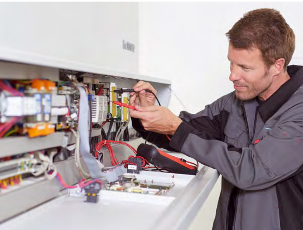
The electrical components are stowed centrally in the wiring cabinet
